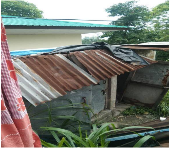
Figure 3: lack of sanitation facilities as captured by a female photovoice respondent in Pasakha, 2024.
