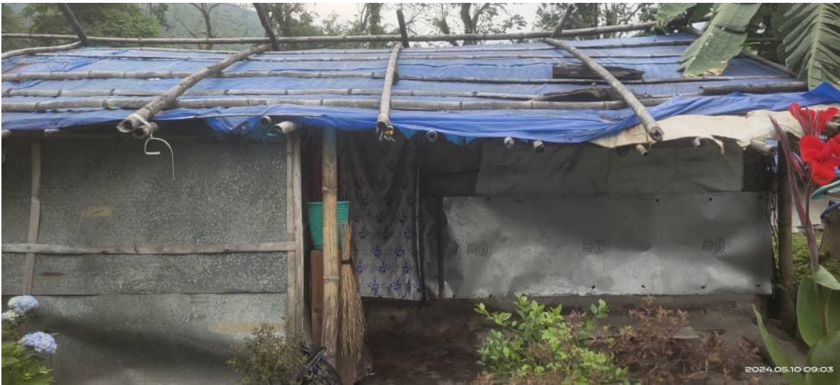
Figure 7: precarious housing conditions in Pasakha. Photo courtesy: photovoice respondent in Pasakha, 2024.
