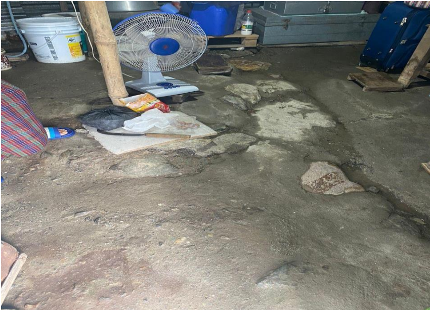
Figure 6: floor of house of migrant worker. During the monsoon, rainwater seeps into the house through the ground. Photo courtesy: photovoice respondent in Pasakha, 2024.
